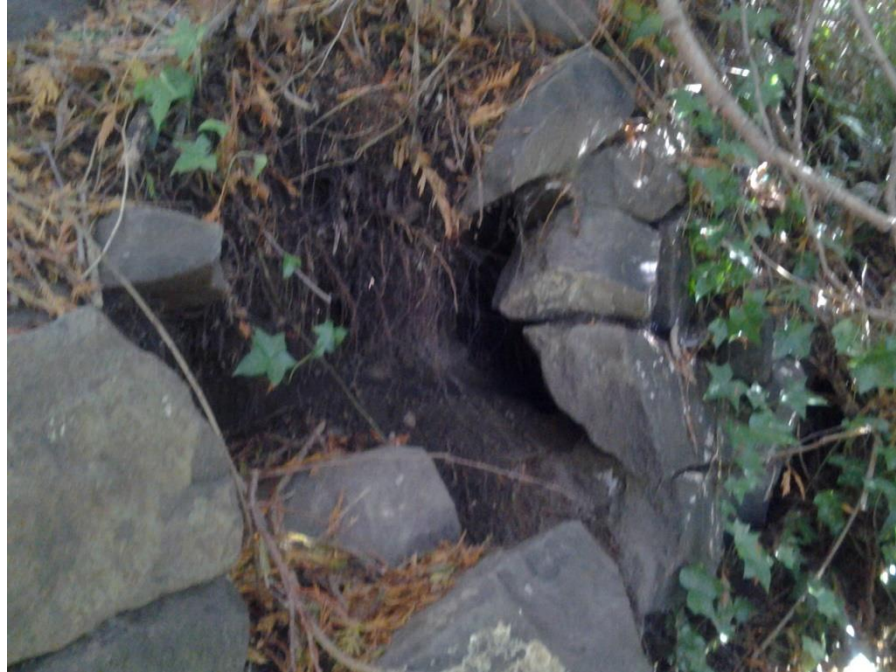
Figure 11. Photo showing one of the locations where the wall is breaking down.
