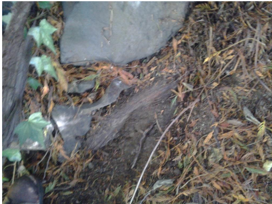
Figure 12. Photo of one of the #10 cedar's roots coming through the wall.
