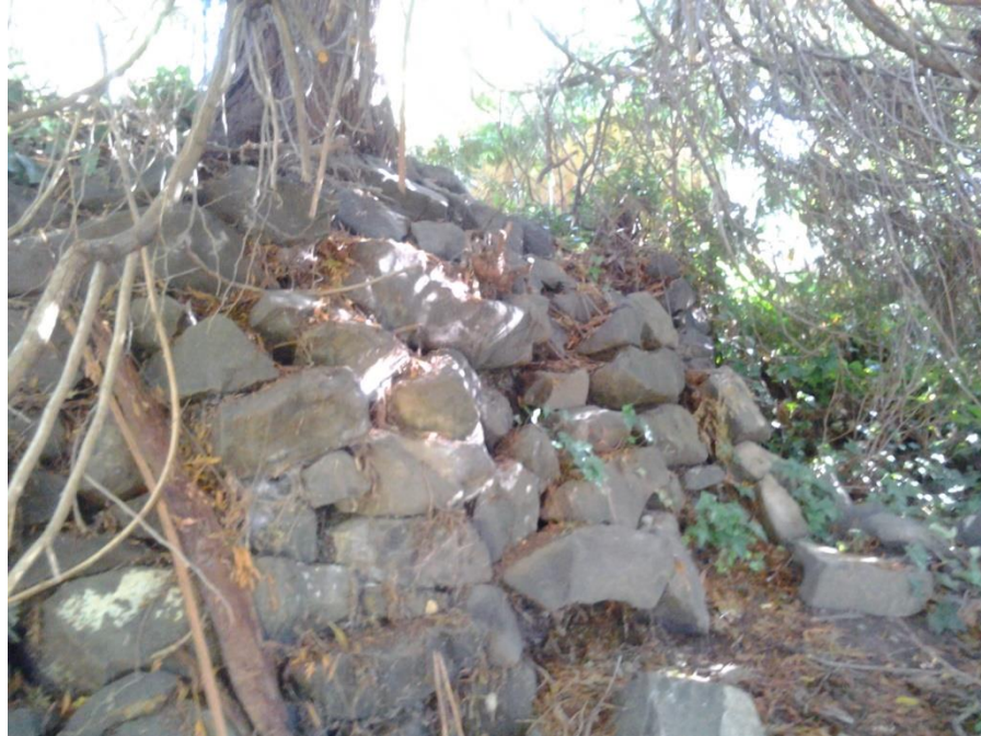
Figure 9. Photo showing the location of the #10 tree at the top of the second rock wall. Note the loose stones scattered at the base of the wall.
